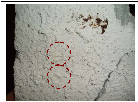
Sealant applied to holes at the stucco subsequent to exterior moisture testing.
