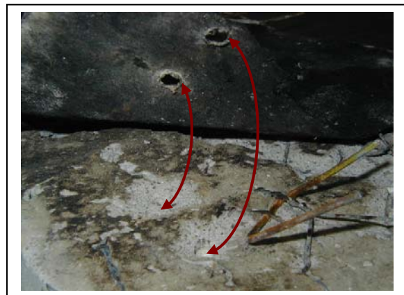
Sealant applied at the stucco subsequent to exterior moisture testing typically does not reach the building paper whereby the drainage plane's integrity is permanently compromised.
